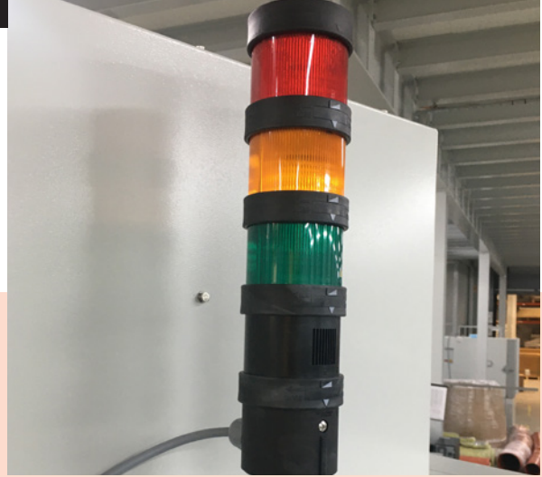
Safety stack light signal
