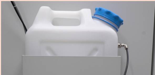
Water supply tank
