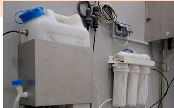
Water Treatment systems
