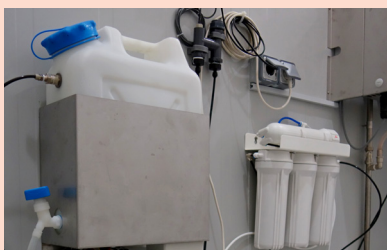
Water Treatment systems
